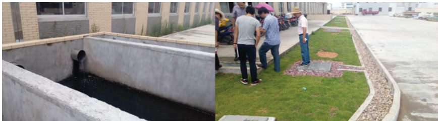
Figure 8.8 Rainwater harvesting system: pre-treatment and storage tank.
